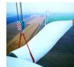
Blade assembly observed from the nacelle.
